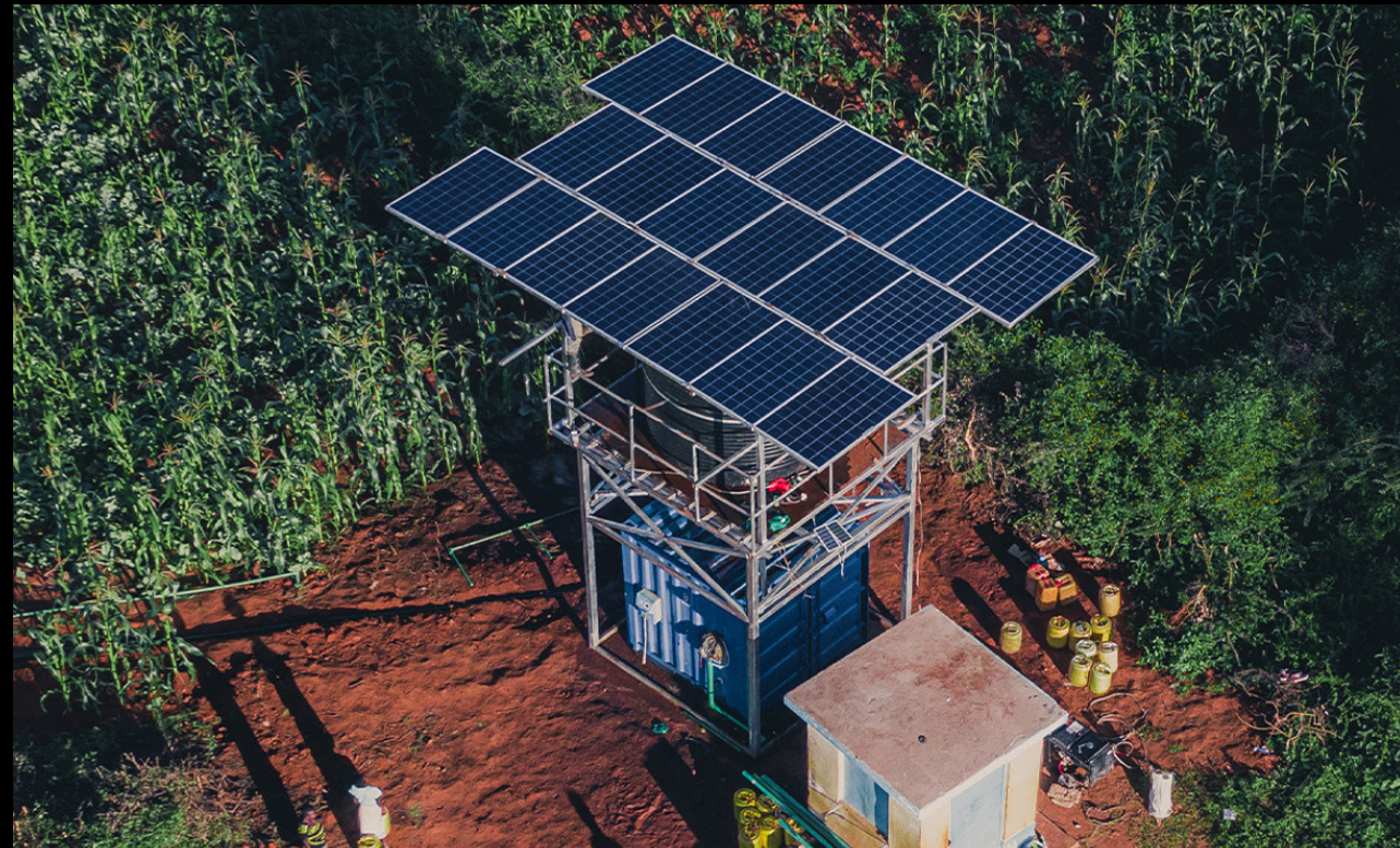
Solar powered water purification
